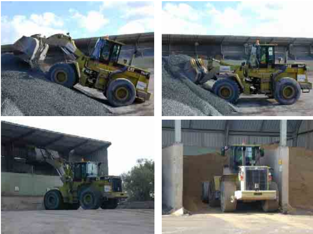
Figure A1.8.1 CAT 950F II articulated loading shovel feeding asphalt plant with aggregate
